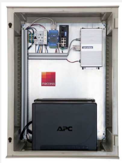
Power Plant Controller
