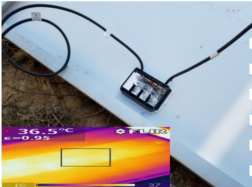
Diode short circuit fault infrared imaging
