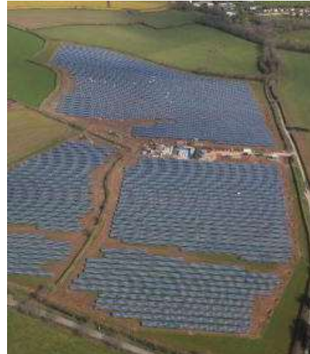
Polos, England Solar Park
